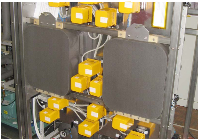
Figure 17. Two Isolated heat exchanger
