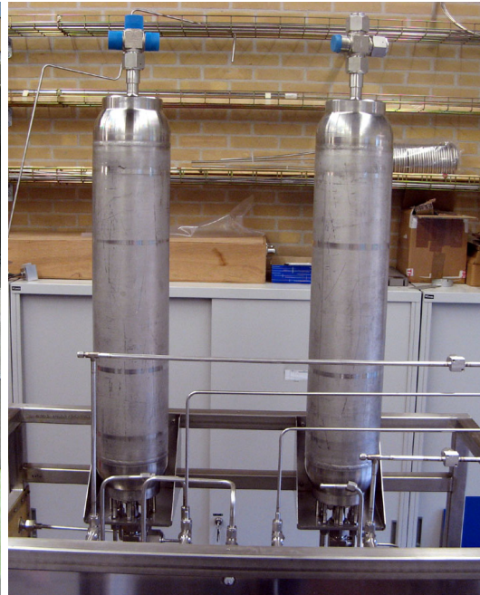
Figure 12. Two accumulators mounted in cooling plant
